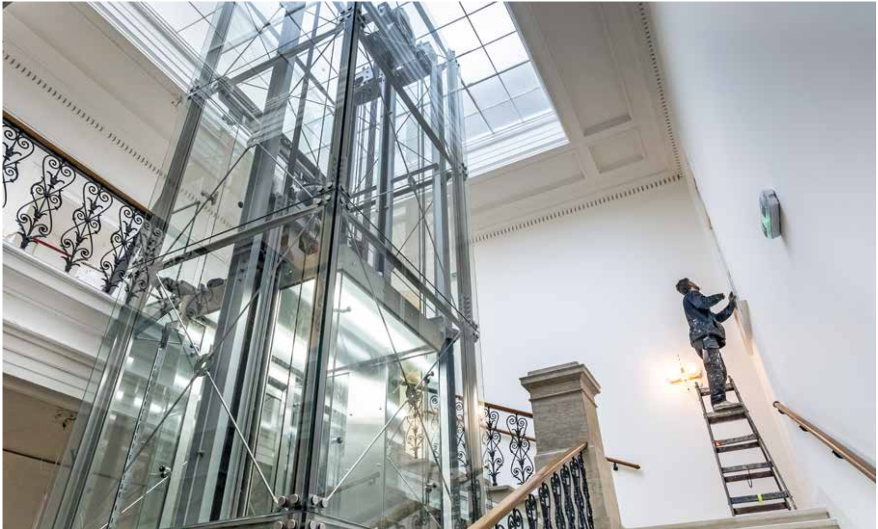
New lift in the north staircase, which was built during the renovation of the staircase in 2021
