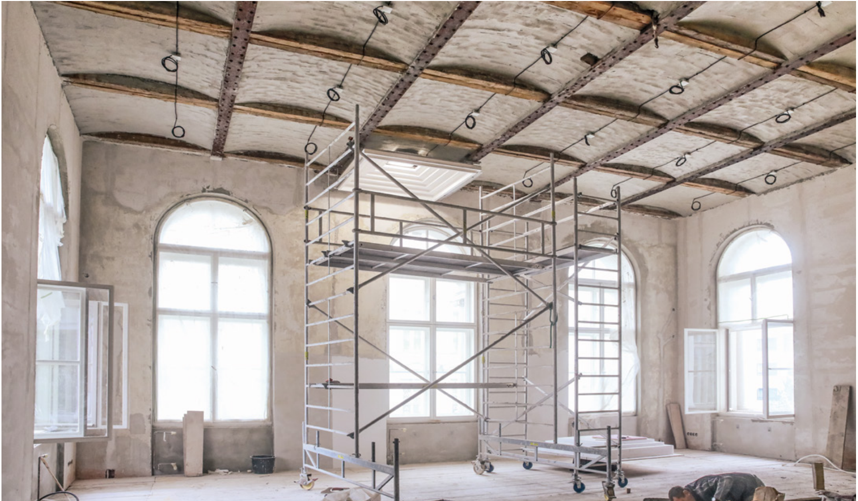
The walls were resurfaced and unfit ceiling parts were removed in the renovation. The picture was taken after trial installation of a ceiling coffer with lighting.
