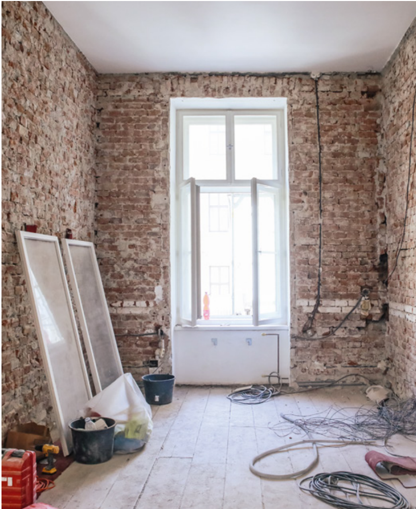
Entrance area for visitors – picture taken during renovation. Unsatisfactory plaster and the upper floor layer were completely removed.
