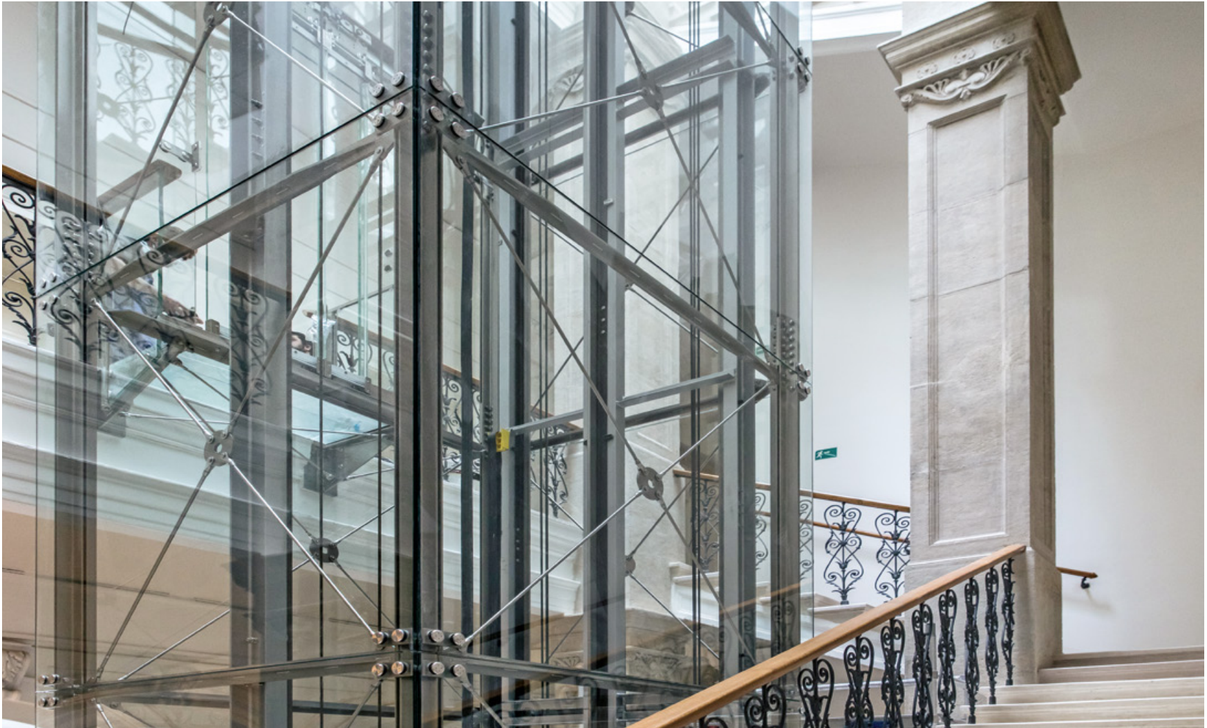
The construction of the new lift was a sensitive matter; the equipment and technology did not disrupt the existing architectural appearance
