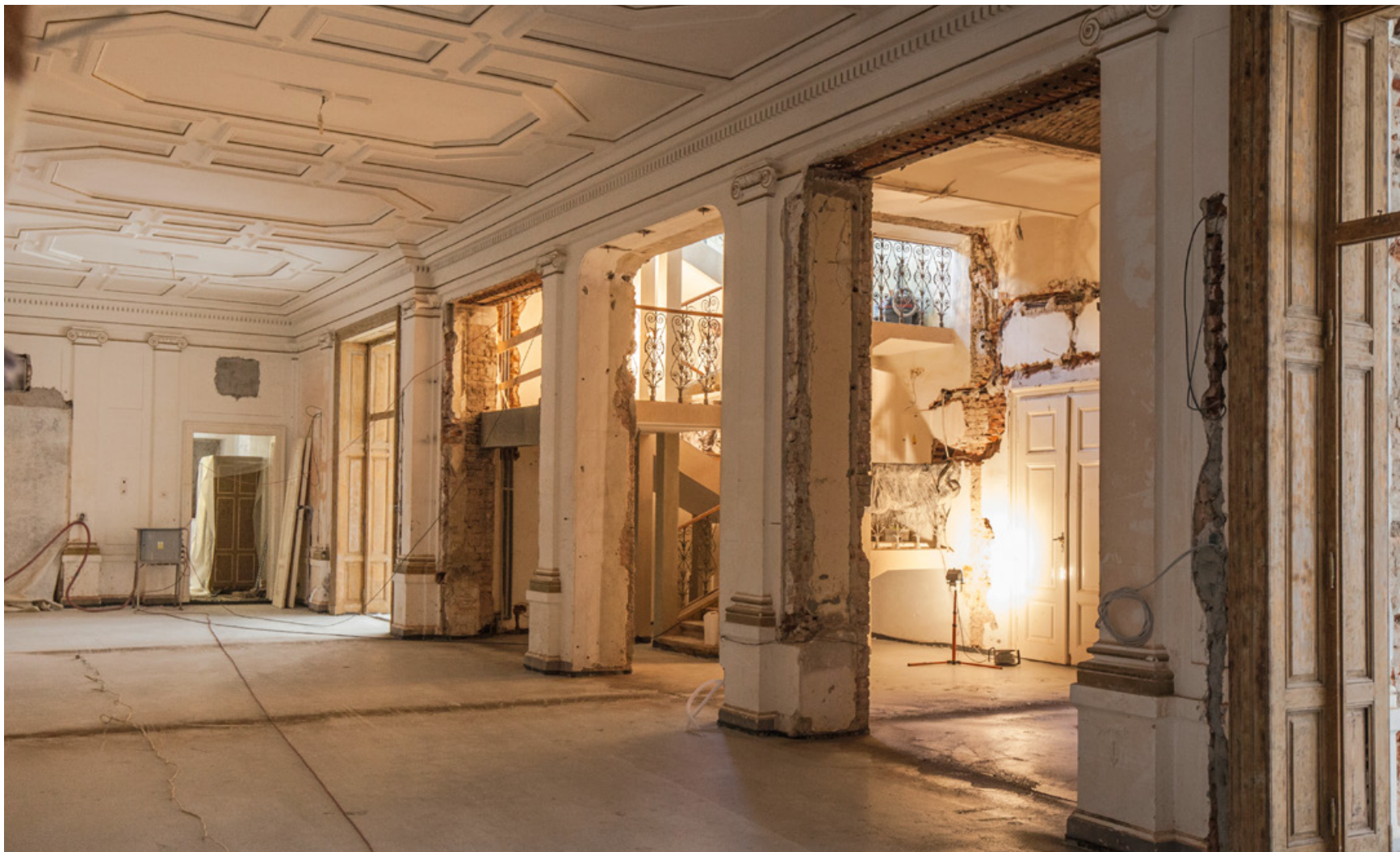
The Vestibul of the Assembly Hall in the course of reconstruction works
