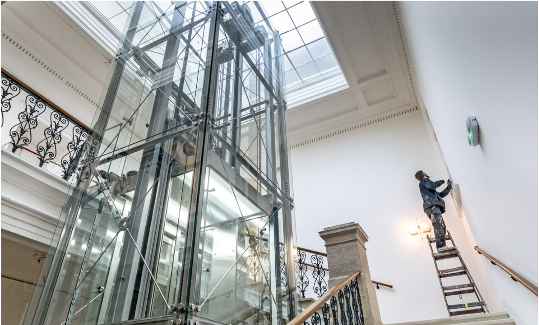
New lift in the north staircase, which was built during the renovation of the staircase in 2021
