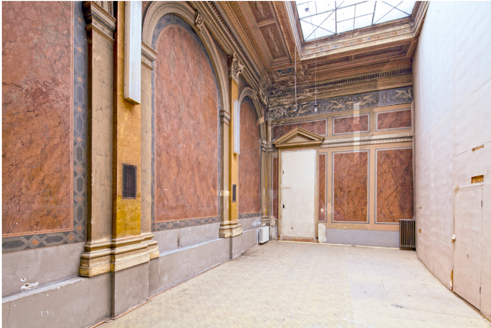
The Western Gallery was not in use due its state of disrepair
