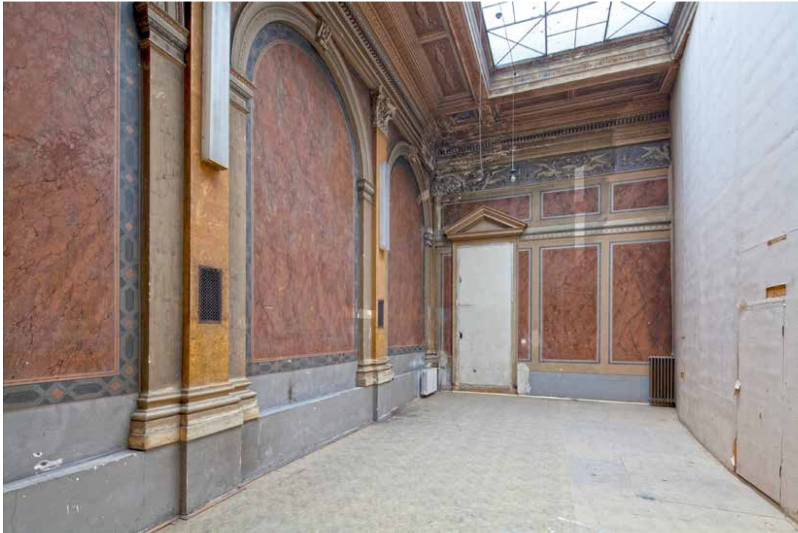
The Western Gallery was not in use due its state of disrepair
